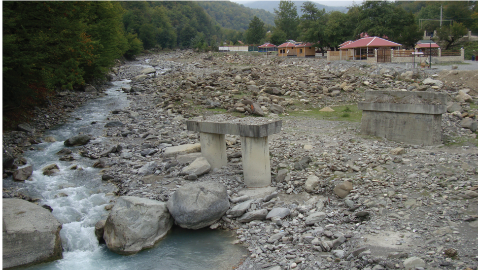
Fig. 1 The bridge over the Shirvanchay River (a tributary of the Goychay River) destroyed on 2 September 2016 by a mudflow in the village of Galajig, Goychay region (photo 12 October 2019)
